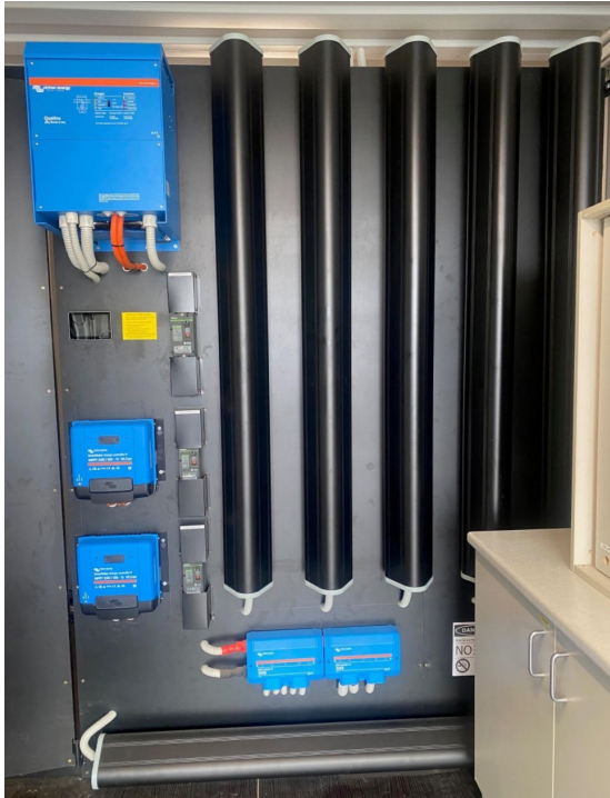
Pictured: Zenaji battery installation at Ray Robson's property.
