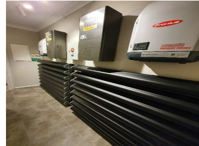
Pictured: Dedicated battery room, installed by Daniel Huppert, with 16 Zenaji Aeon batteries.
